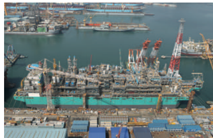
PFLNG Satu , the world's first floating LNG production (FLNG) vessel, under construction
